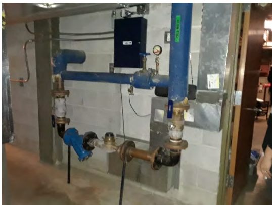
Birch Bldg. Domestic Cold Water Service
