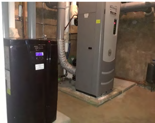
Birch Bldg. Dom Hot Water Heater & Heating Boiler
