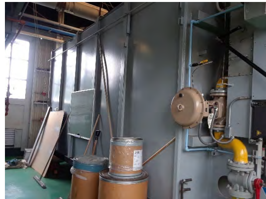
Existing Spring Boiler
