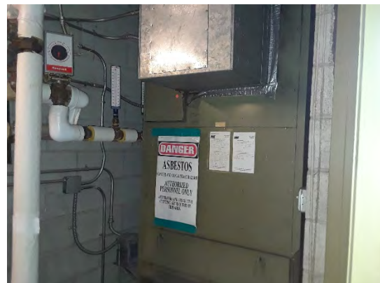
Ventilation Heating Unit
