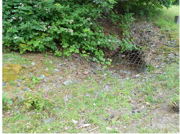
PORTION OF HAMLIN CREEK IS IN OPEN DITCH ALONG EAST PROPERTY LINE
