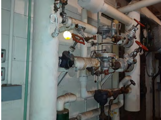
Steam Pressure Reducing Station
