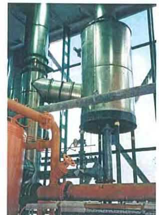
Installation of a DC-2-300 SUPERMIZER servicing a 300 HP. Fulton Hot Oil Boiler. Note simple support frame eliminates structural roof support members
