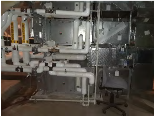
Birch Bldg. Air Handling Units
