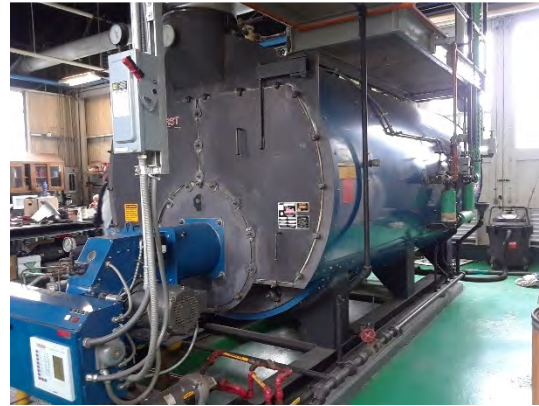
Existing Summer Boiler
