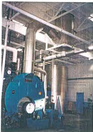
Installation of a DC-2-500 SUPERMIZER servicing a 500 H.P. boiler.
