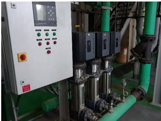
Existing Boiler Feed Pump Set
