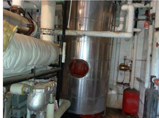
Dom Hot Water Heater
