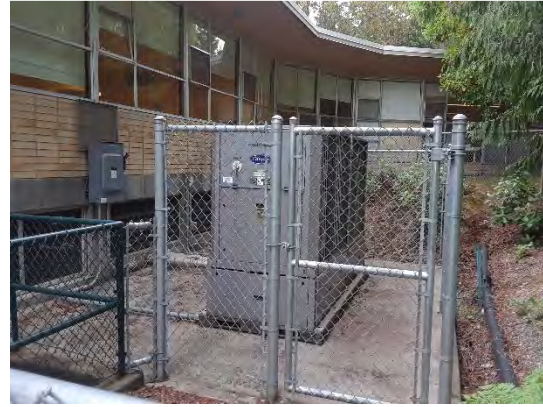
Birch Bldg. Air Cooled Chiller
