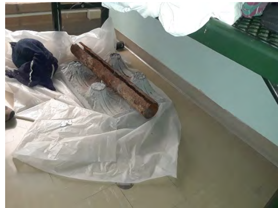
Birch Bldg. Corroded Waste Piping and Piece of Floor Slab
