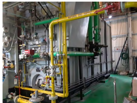
Existing Summer Boiler
