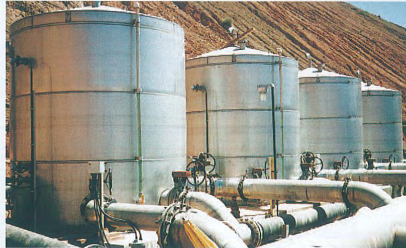
Four of sixteen 12,000 gallon T-316L stainless steel tanks for acidic leach solution in mining operations for Bechtel Corp.
