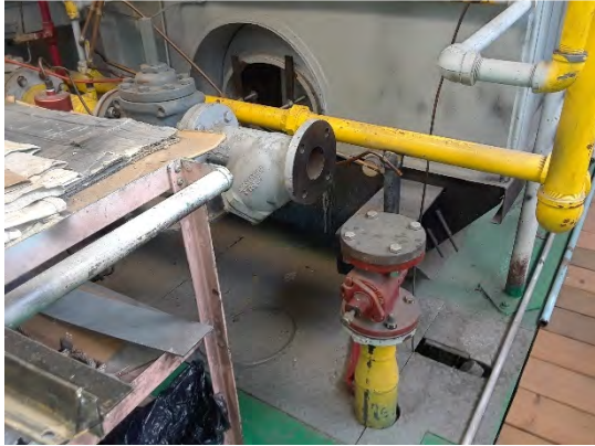
Disconnected Abandoned Boiler
